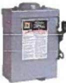
Photovoltaic AC Disconnect
